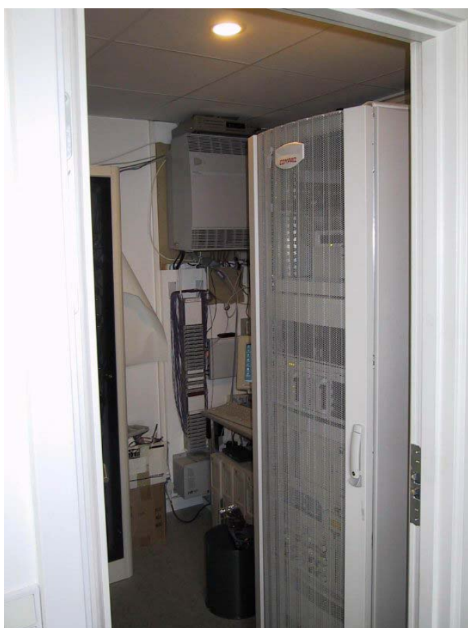
Figur 4. Rack'et i serverrummet.
