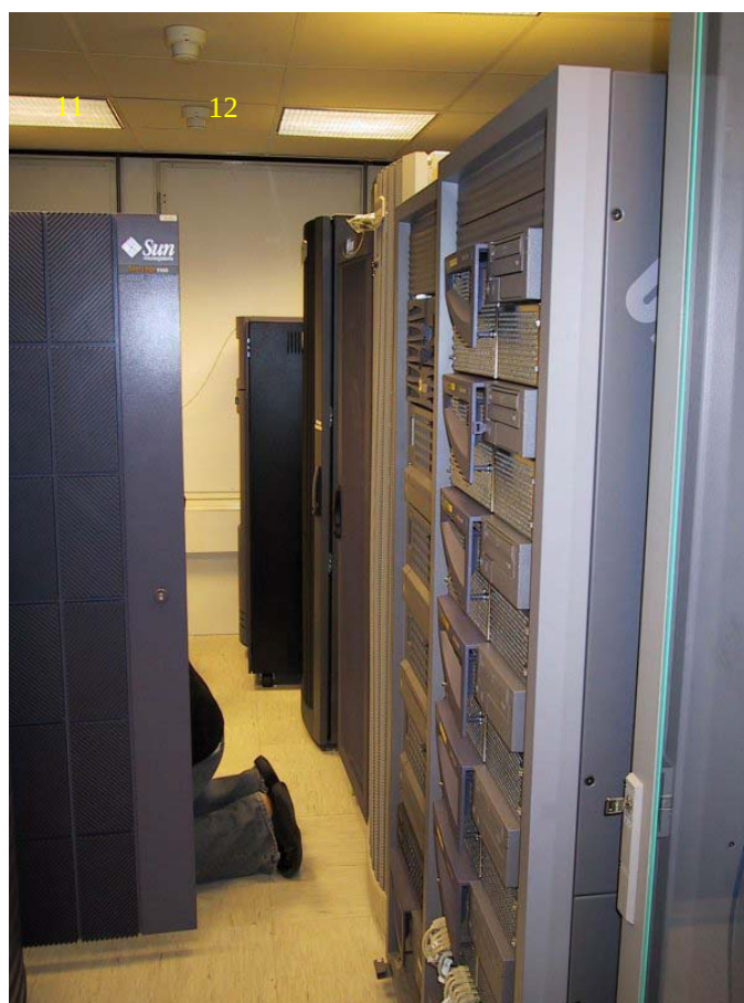
Figur 5. Rack'ne i serverrummet.
